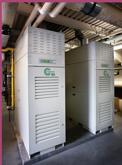
Capstone C65 microturbines
