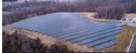
Mill Road - 18 MW
