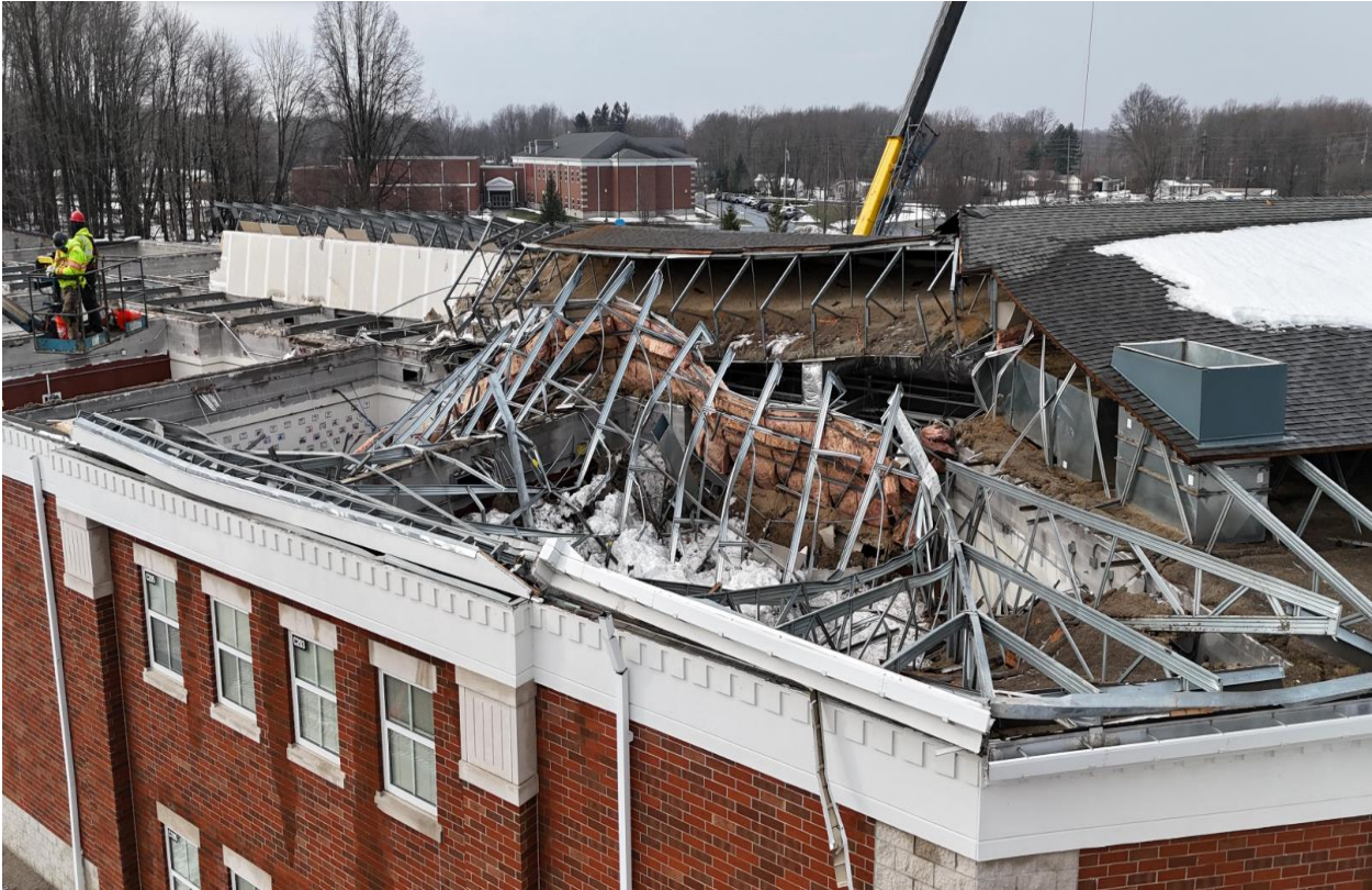
Exhibit 4 – Collapsed Roof being removed
