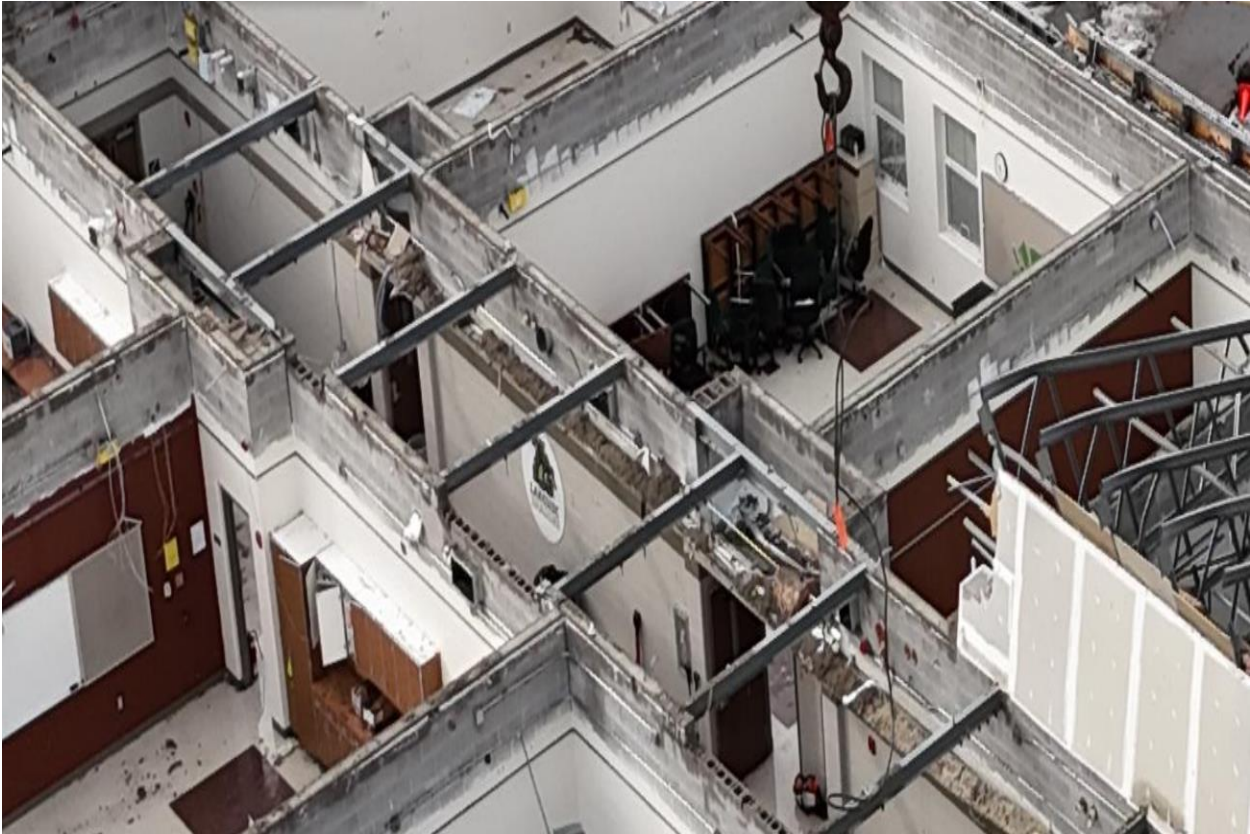
Exhibit 3 – Support walls – Concrete walls on upper floor are compromised and need to be further looked at.
