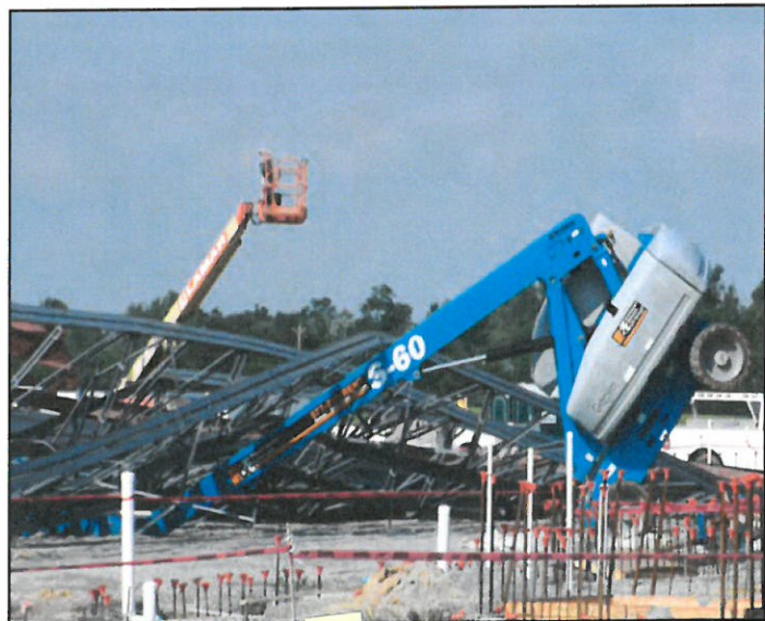
Uppedended Construction crane— McCracken County Collapse
