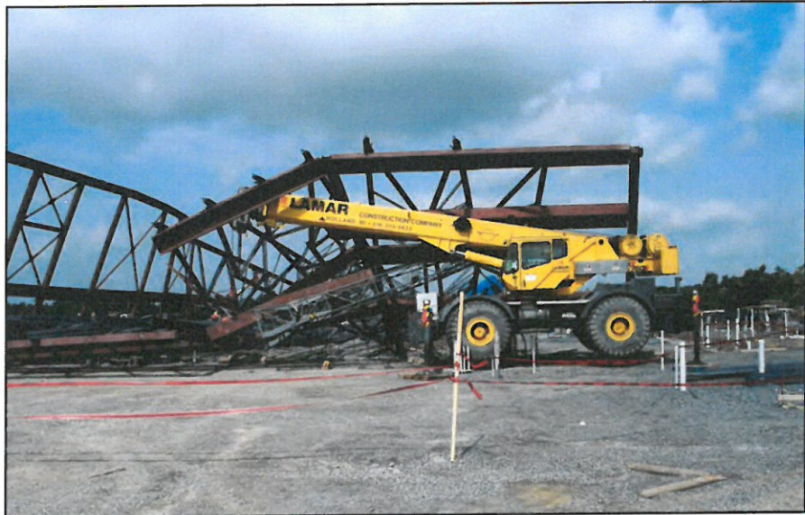
McCracken County Consolidated High School collapse May 22, 2011. Construction provided steel erection & welding services on the project
