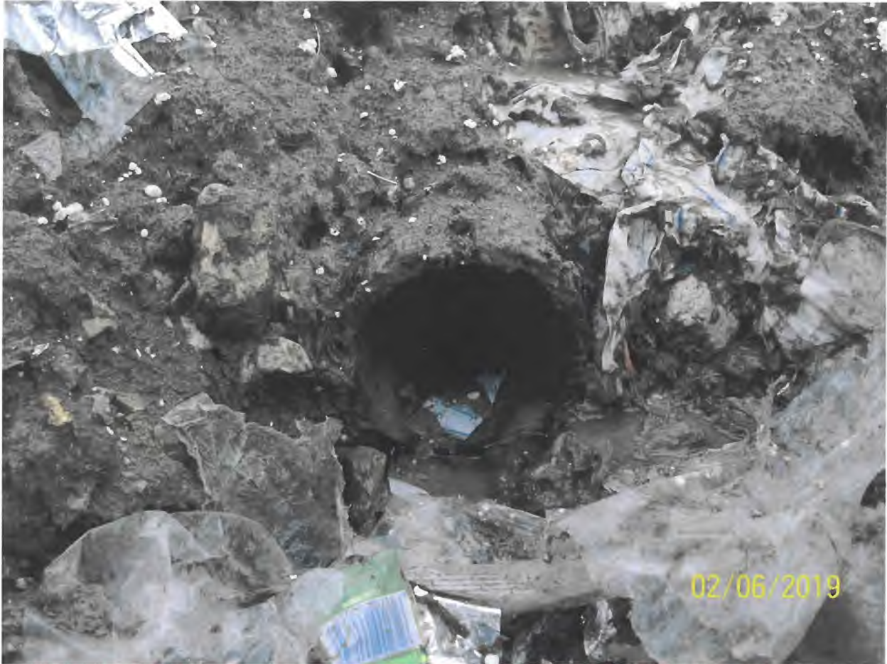
6) Outlet end of the drain pipe as it daylights along the western edge of the east pond.
